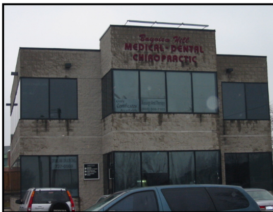
Figure 1. Rain wetting pattern on building cladding
